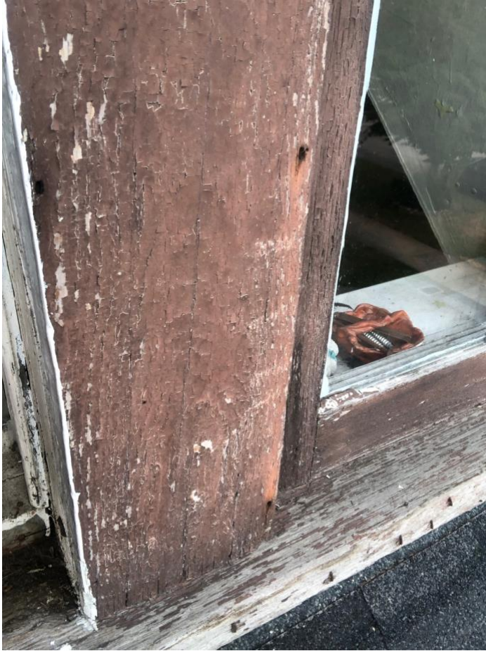
Figure 18c: Attic dormer window, sill and trim – north side.
