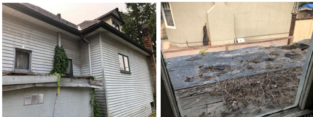
Figure 19a: Soffits and gutters on the north side, deteriorated roof covering storage area on north side
