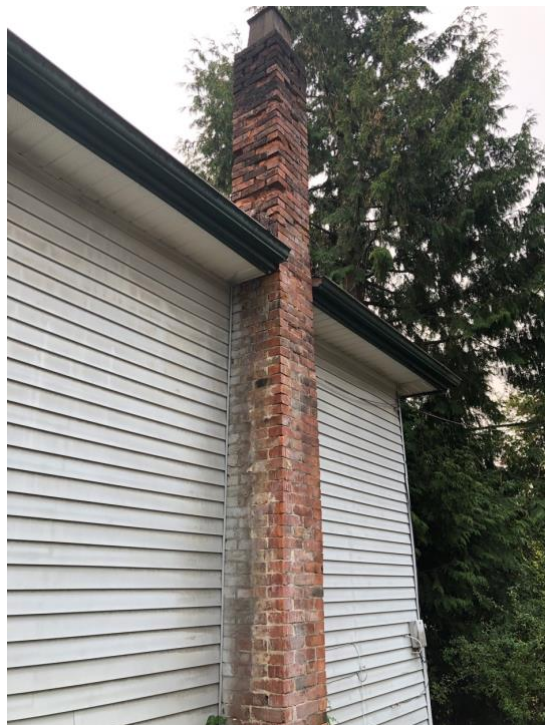
Figure 20: Deteriorated chimney on north side
